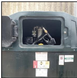
Bunded oil tank with a lockable hatch
